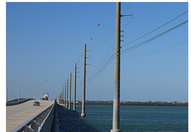
Hundreds of concrete utility poles require capping to prevent corrosion
